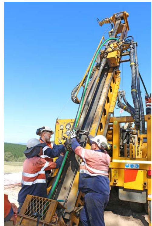
Figure 1 - The drilling crew completing the casing of Hole #1 with high pressure polyethylene pipe on Thursday 5 February.
